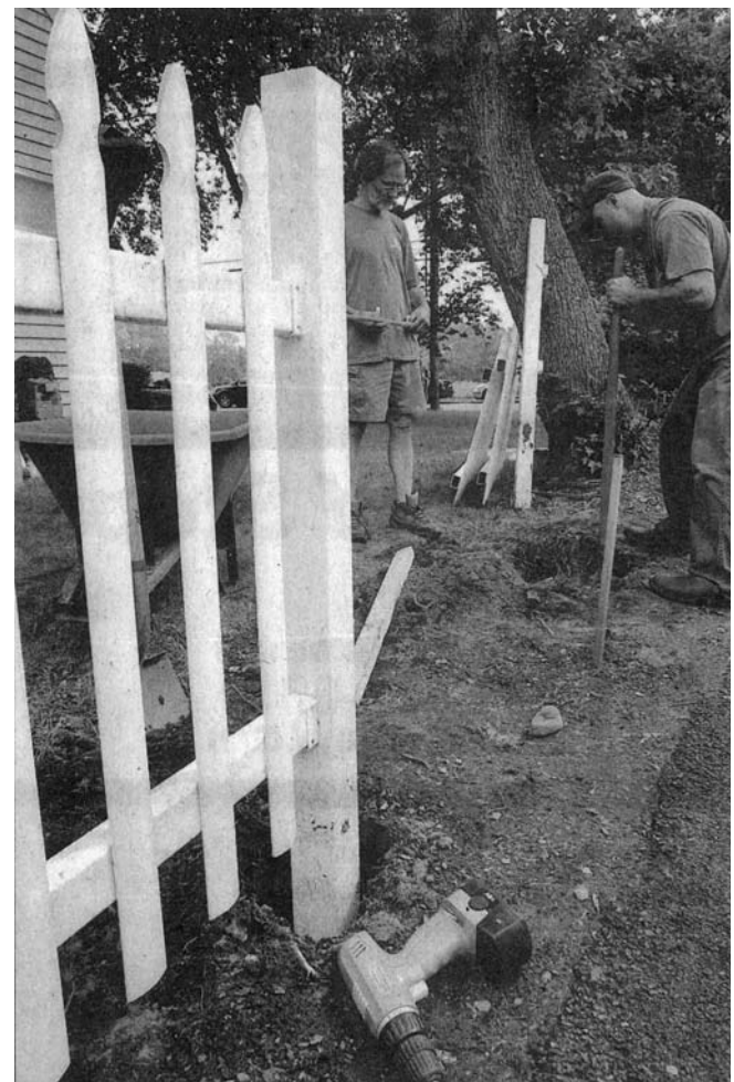
Jay Hart left, and Nick Coufas dig post holes for a fence that will surround a vegetable garden for Tina Vitale.
